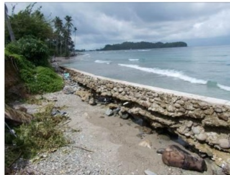
Fig. 1 Ground scour behind the revetment building due to overtopping waves
